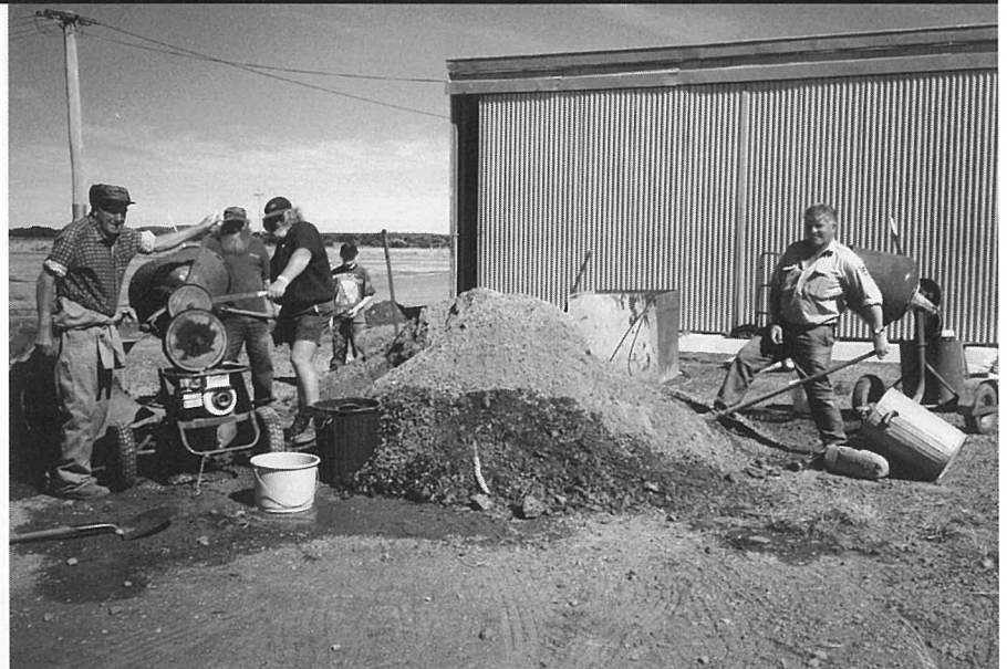
Club members from Bishopsbourne, NTFA and FACT, and PWS officer laying the foundations The new shed - completed by May 2000
